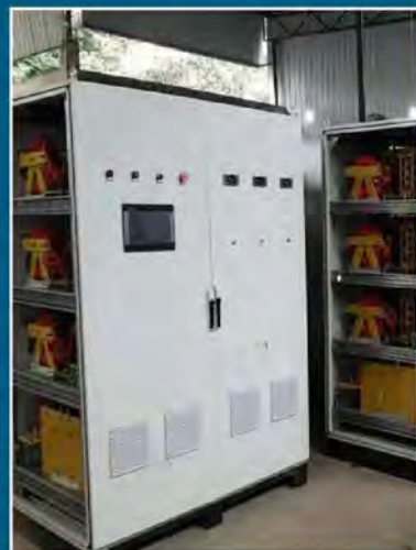
电源柜 Power cabinet
