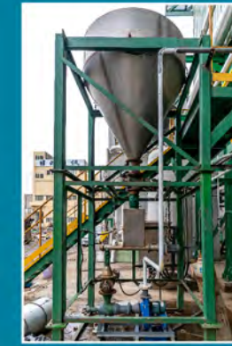
活性炭输送系统/ Activated carbon conveying
